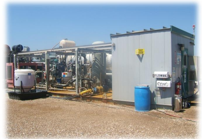
Fountain Quail MVR NOMAD Facility ALL Consulting
